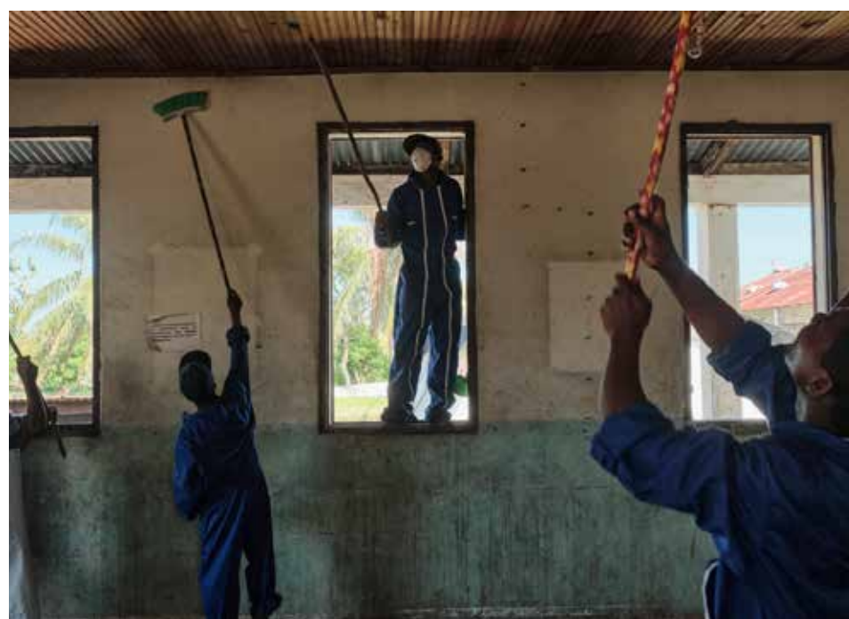
MADAGASCAR: A hospital in Nosy Varika is cleaned and rehabilitated after being partially destroyed by cyclones. MSF teams supported the hospital's medical activities and rehabilitation, as well as five other health centers damaged by the cyclones in this remote area. 2022 © iAko M. Randrianarivelo/Mira Photo
